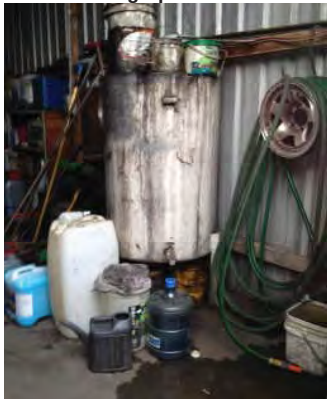
View of the above ground oil tank
